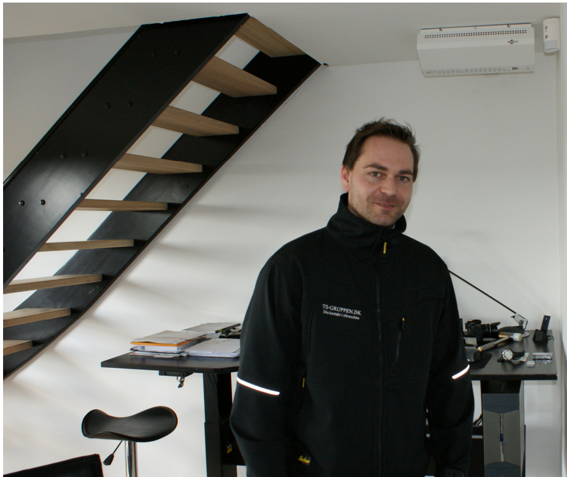
Fog security in a private home. The fog cannon to the upper right was installed by Per Kilsmark Rasmussen of the VS Automatic alarm company.
